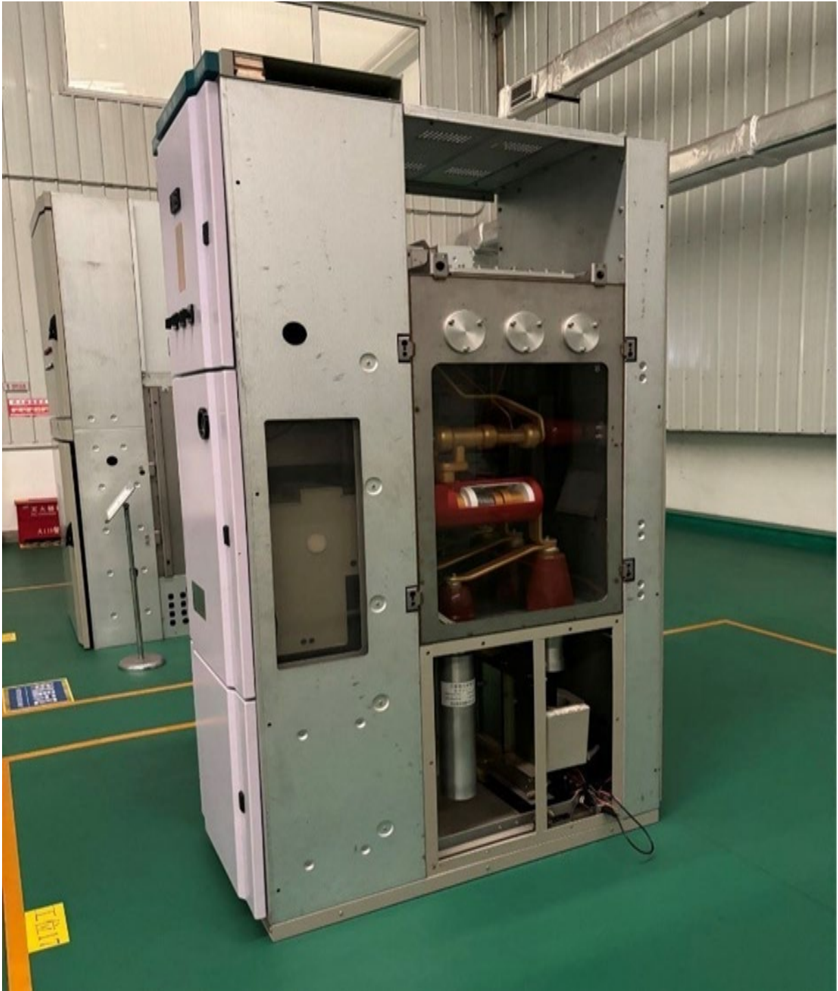
Fig. 3 .INSIDE VIEW OF HG4-12 12KV Rated CGIS , 630A , 20kA/3 sec
