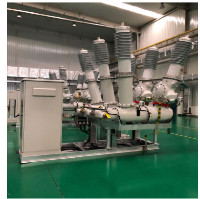
72.5 Kv Outdoor switchgear
