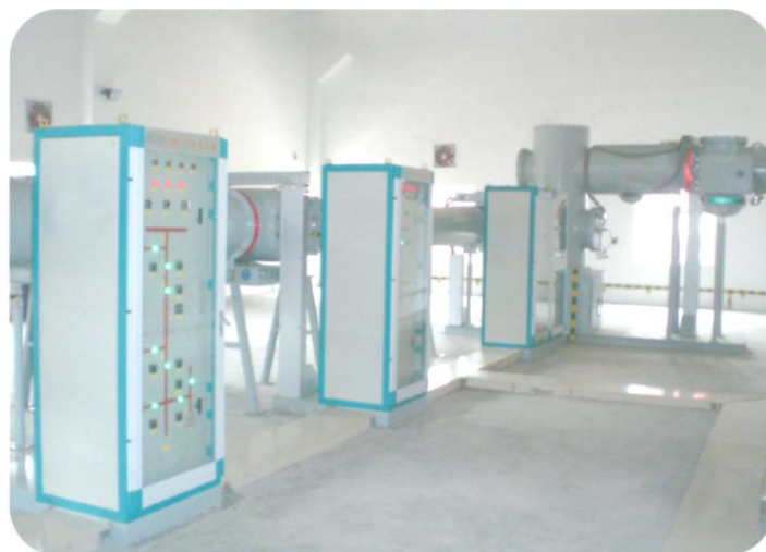
Control panel in operation
