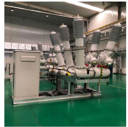
72.5 Kv Outdoor switchgear
