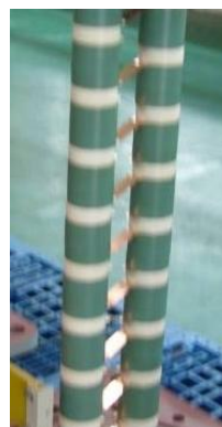
Zinc oxide valve
