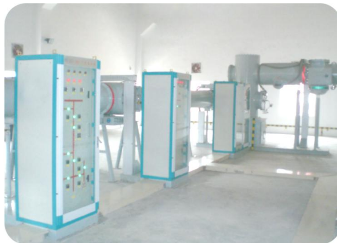
Control panel in operation
