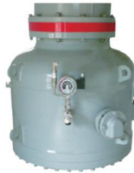
Voltage transformer (VT)
